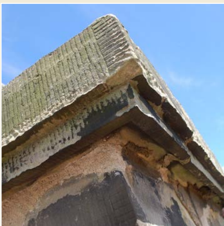
Fig. 9 A chimney cope showing the drip detail to the underside, designed to shed water.
