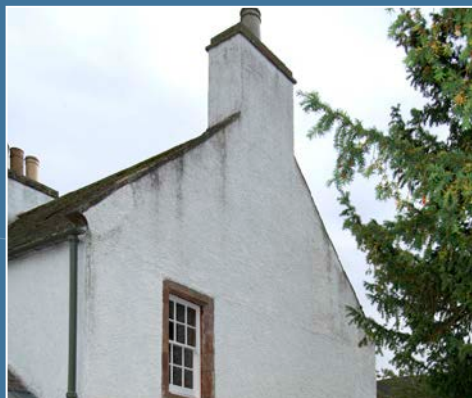
Fig. 1 The gable end of a traditional building showing signs of staining caused by water run-off.
