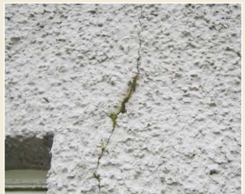
Fig. 5 Moss growing in a crack in cement roughcast, indicating wet masonry behind.
