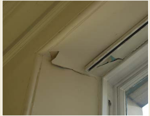
Fig. 3 Damage to internal finishes as a result of dampness caused by a defective cornice on the external masonry.
