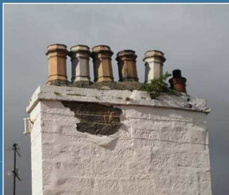
Fig. 2 The poor condition of this chimney is likely to cause problems to the gable below.
