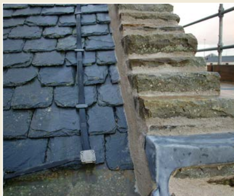
Fig. 13 A mortar skew fillet, which forms a weathertight seal between roofing slates and masonry.
