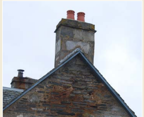
Fig. 4 Salt staining in saturated masonry caused by a chimney in poor repair.
