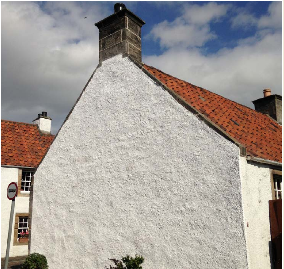
Fig. 16 This gable end is drying out following repairs and improved detailing at the skew copes, and the application of traditional harling and limewash.
