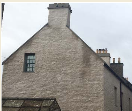
Fig. 15 Dampness persists on new harling due to inadequate detailing on the skew copes.
