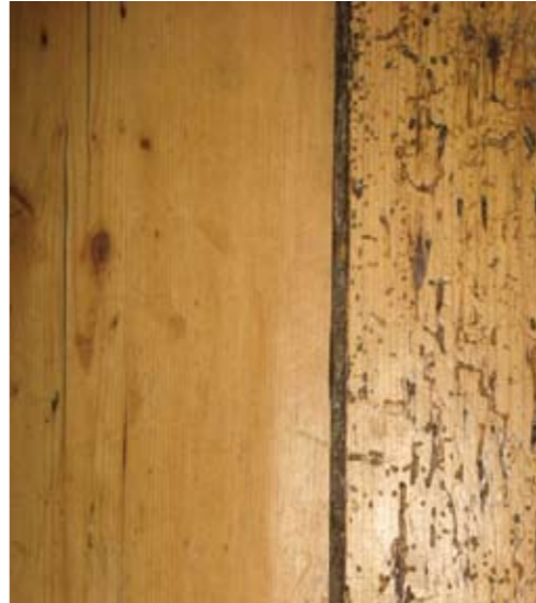
19th C flooring, showing wood beetle attack (no longer active) on the softer timber.
