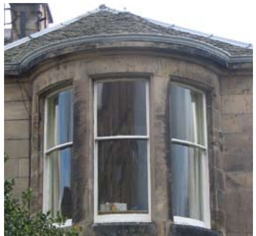
Curved glass can be difficult and expensive to replace
