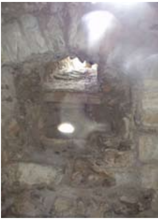
Water inlet and outlet
