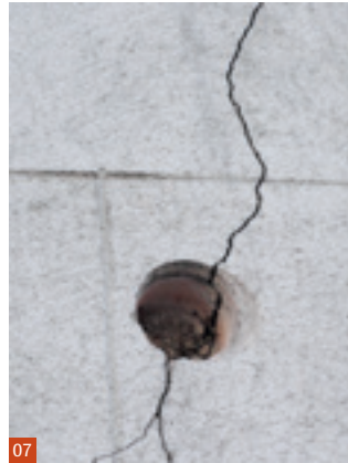
Fig. 6 Shrinkage cracks in a mass concrete wall, built c. 1880.
