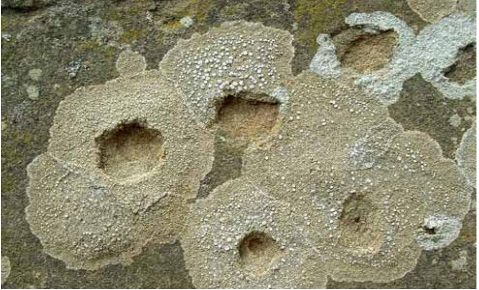
Fig. 4 Rare example of damage to sandstone masonry caused by lichen growth.
