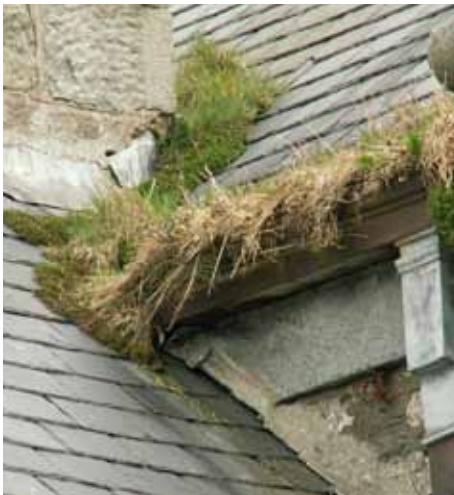
Fig. 5 Guttering clogged by plant growth.
