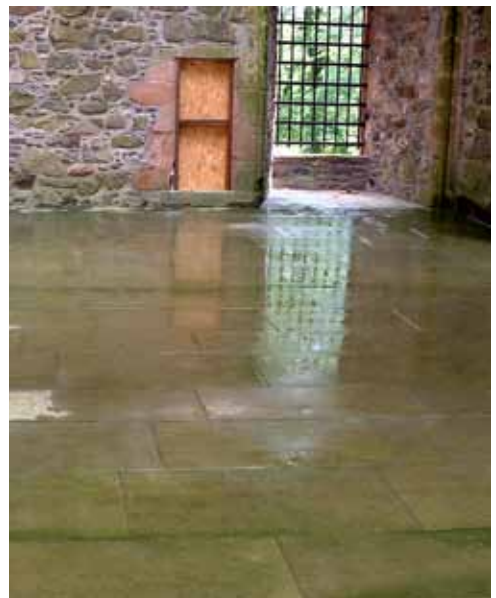
Fig. 3 Slime producing algae may result in slippery surfaces.
