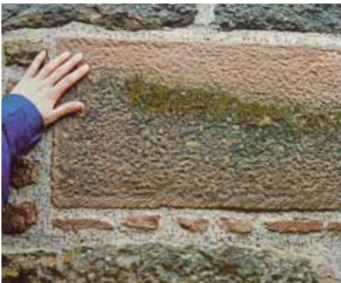
Fig. 2 Inhibited biological growth due to alkaline conditions caused by new mortar.
