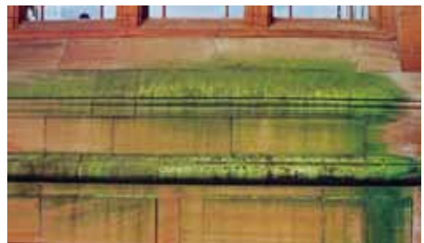
Fig. 6 Rapid re-colonisation by algae of a recently cleaned sandstone building.
