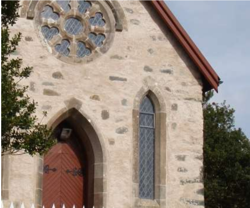
Fig. 2: Detail of the lime pointing on the west gable; this resulted in much drier masonry
