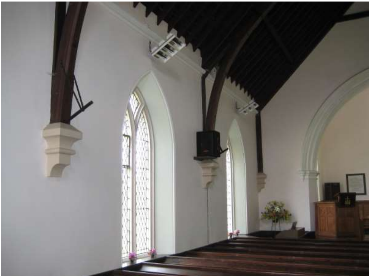
Fig. 3: Hobkirk Church in the Scottish Borders is heated by radiant panels at cornice level
