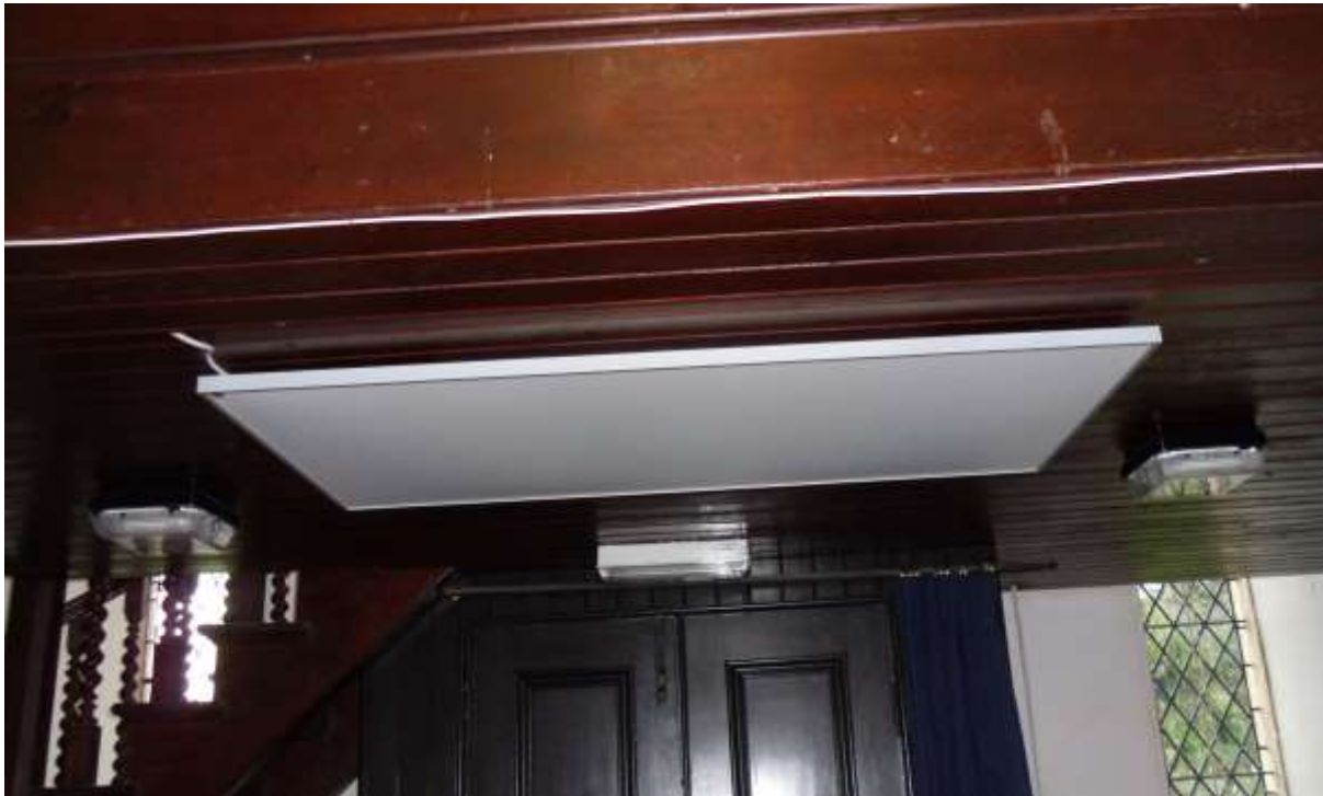
Fig. 6: The radiant panels underneath the mezzanine layer
