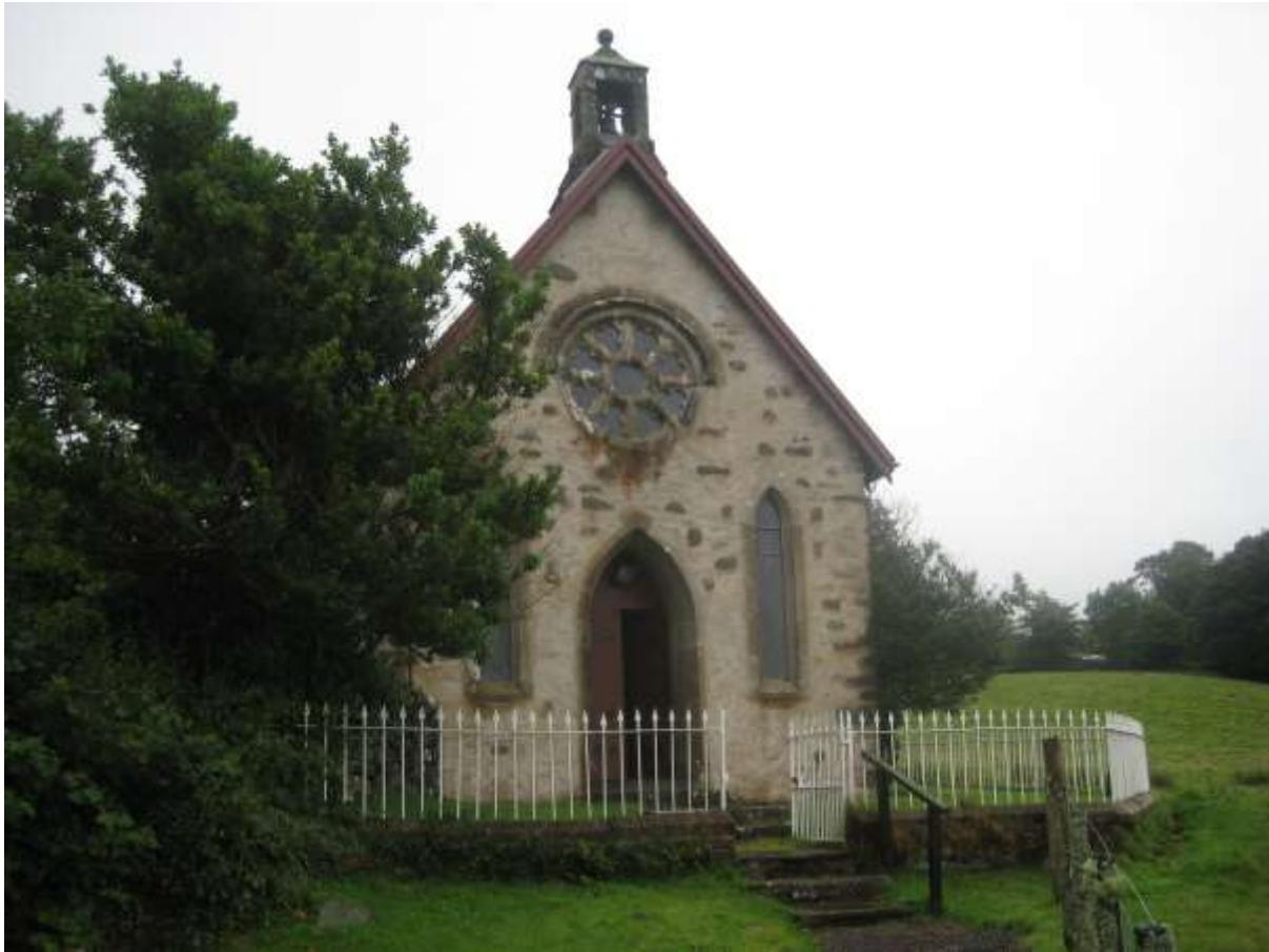
Fig. 1: Kilmelford Church viewed from the West; the lime mortar repairs to this elevation were an important first stage in the building upgrade
