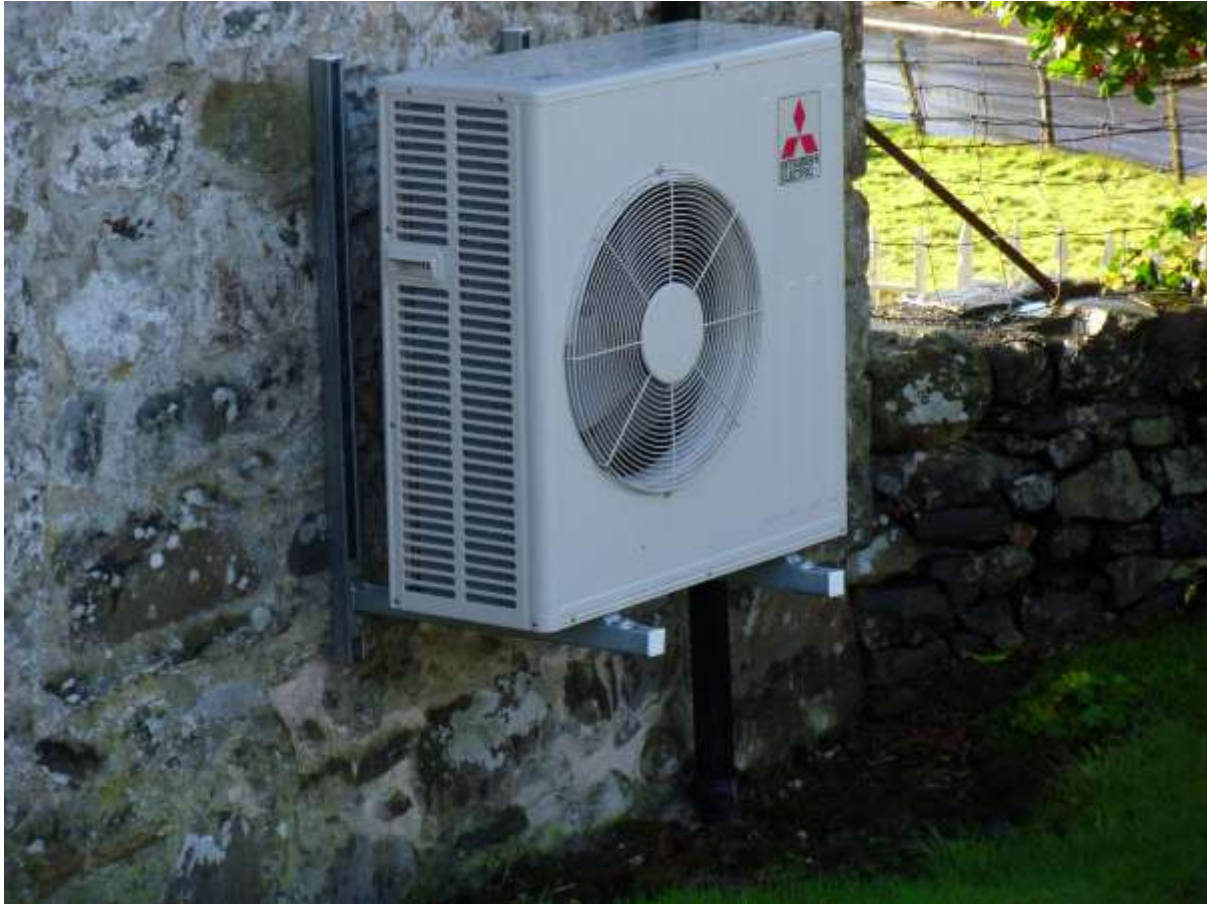
Fig. 8: The external fan unit of the ASHP on the NW corner of the church
